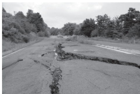
Damage caused by earthquake
